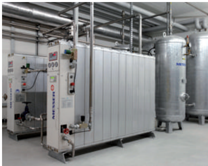
PSA unit for the production of nitrogen
