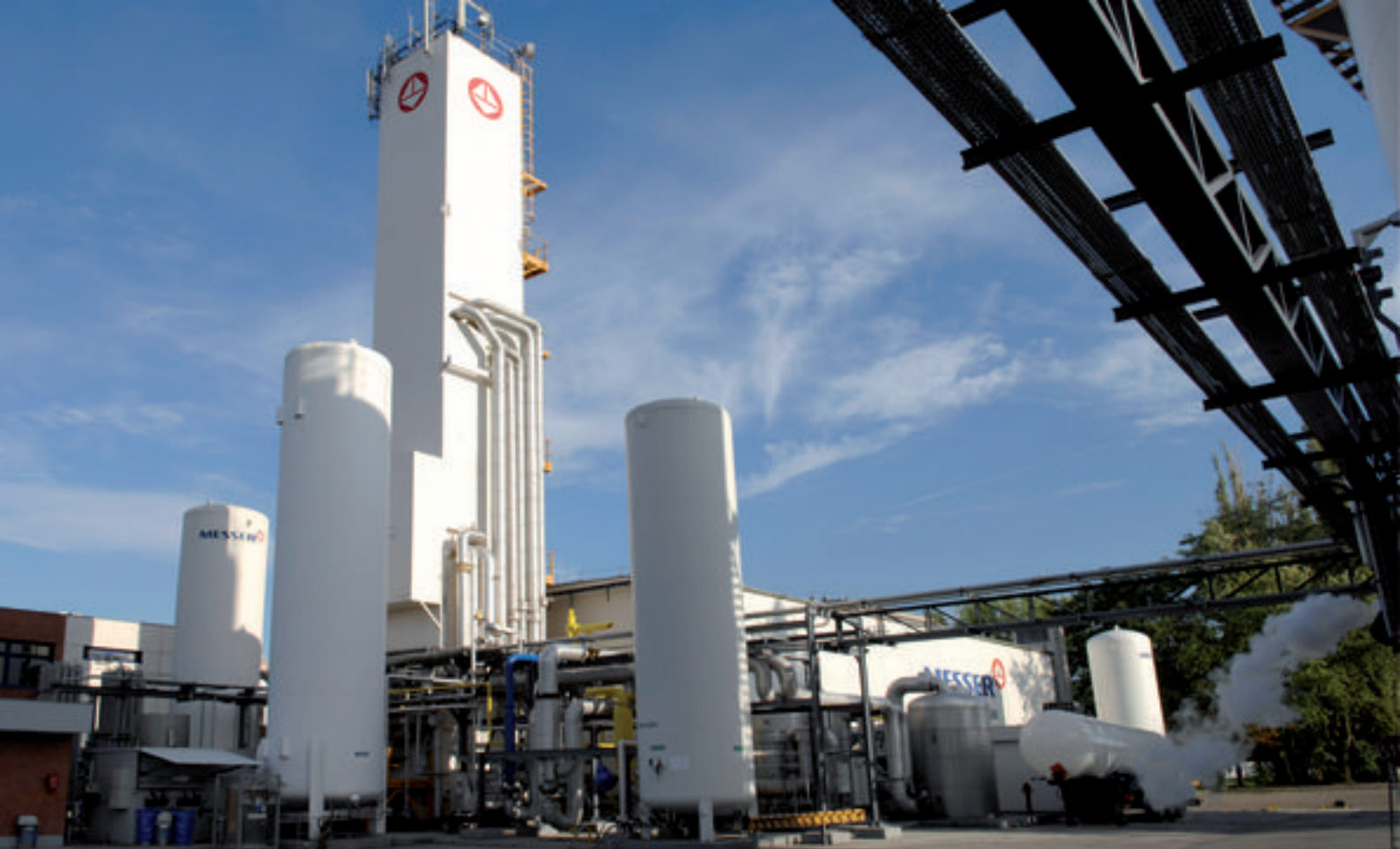
Air separation unit at Messer in Hungary
