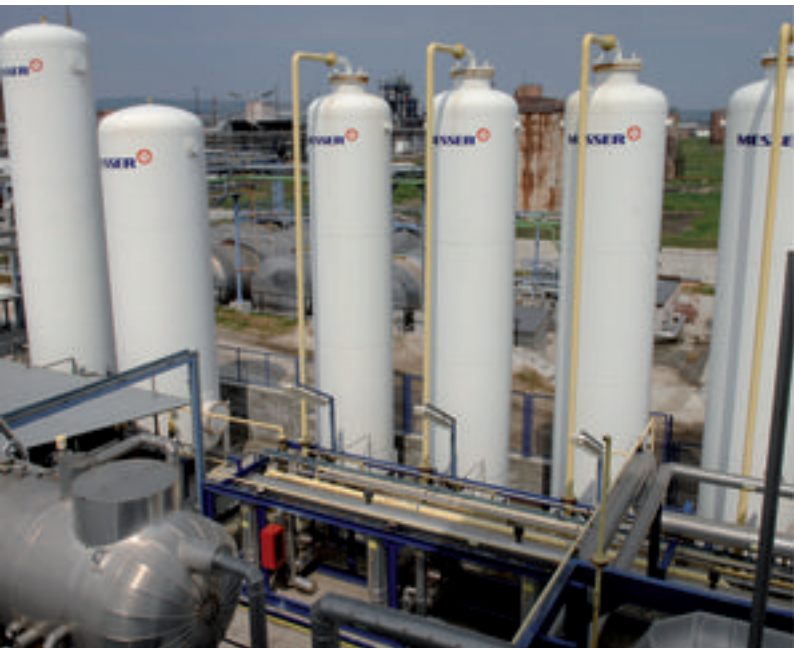
PSA unit for hydrogen production
