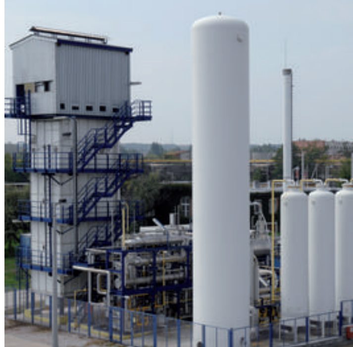
Hydrogen unit, 2,000 Nm 3 /h
