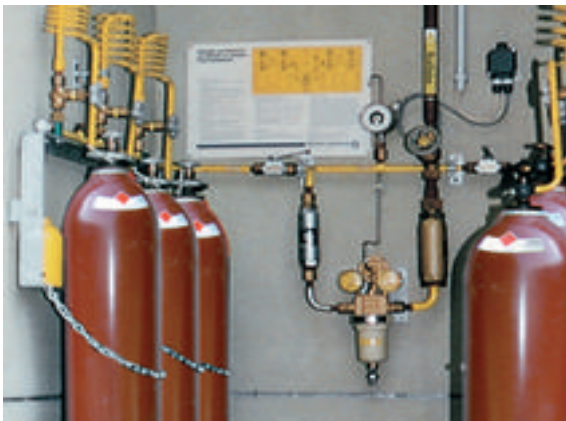
Switchable cylinder bundle station
