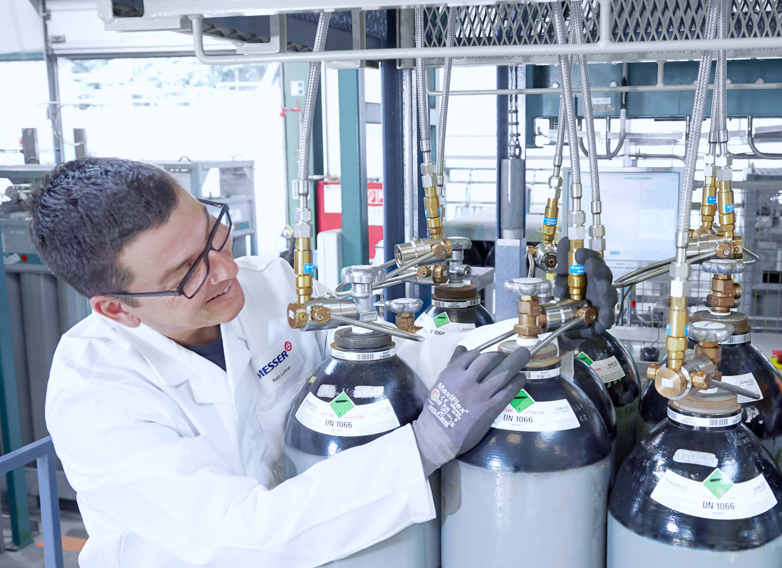
Filling station for high-purity gases
